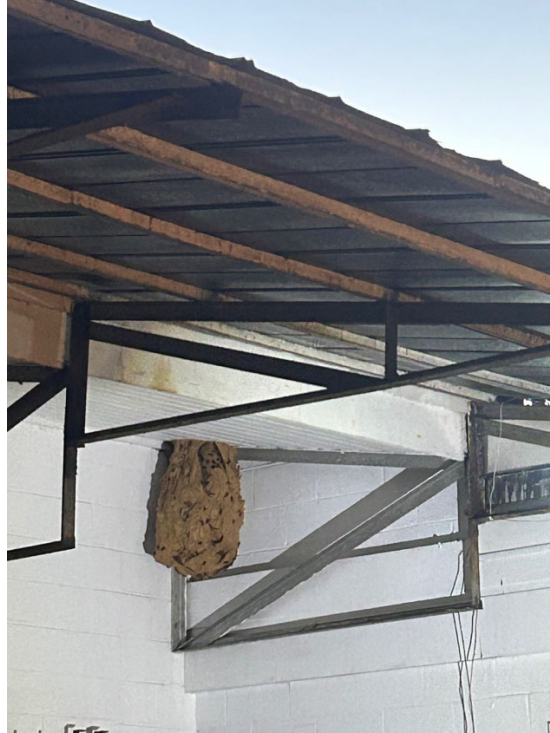
A large YLH nest found by the PPD team under a carport in the Sandfly area of Savannah. (Photo by GDA)
